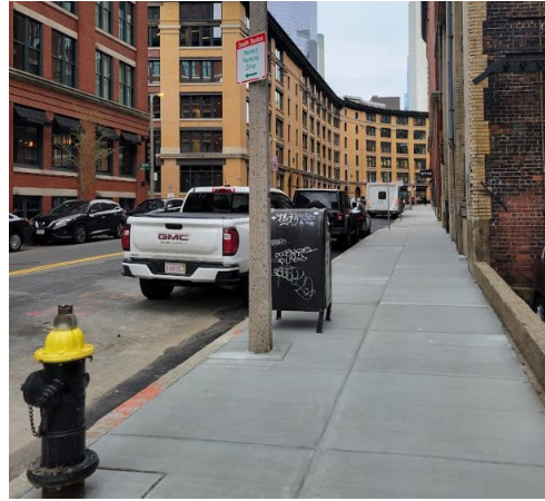
Reconstructed a section of curb and sidewalk on Melcher Street, creating new on-street RPP spaces to offset parking removed on A Street.
