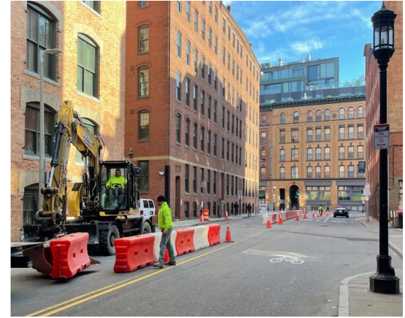
Set up the work zone on the North side of A Street and began curb and sidewalk work.
