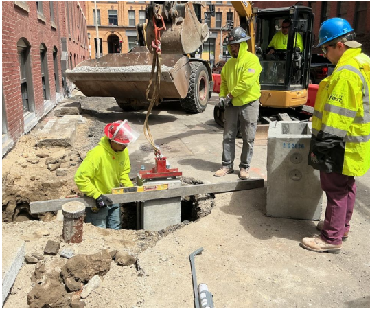
Relocated and installed new drainage infrastructure to make room for the widened sidewalks on A Street.
