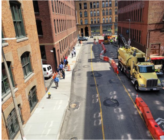
Completed sidewalk work on the North side of A Street, and flipped the work zone to the South side.
