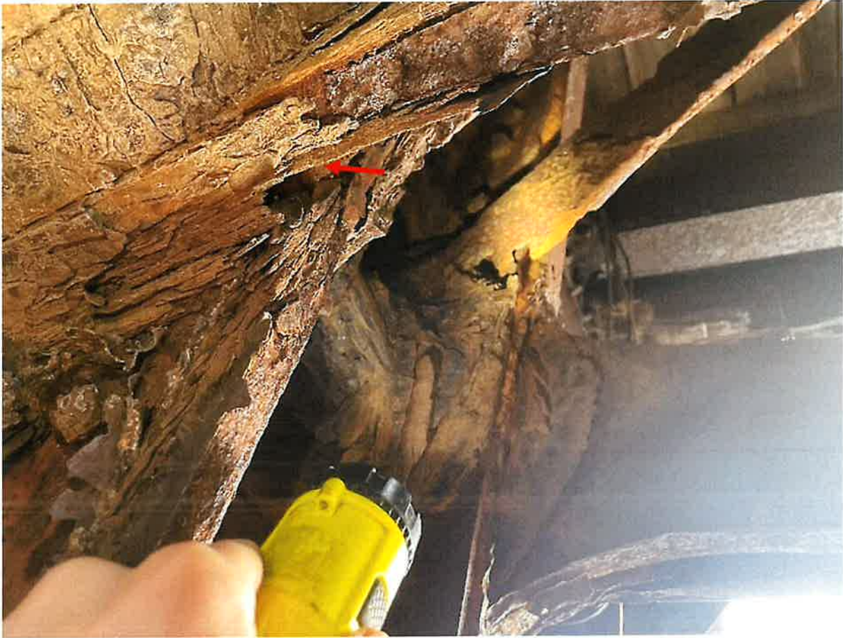
Photo 5. Span 2, North Truss, Diagonal, L26-U27 (Looking Northwest) The north diagonal bar has a 3" W x 3" H rust hole at the bottom with 1-1/2" for the remaining width. The south diagonal bar has 1/4" average remaining by full width. If the north diagonal bar fails, the south diagonal bar will have torsional forces.
