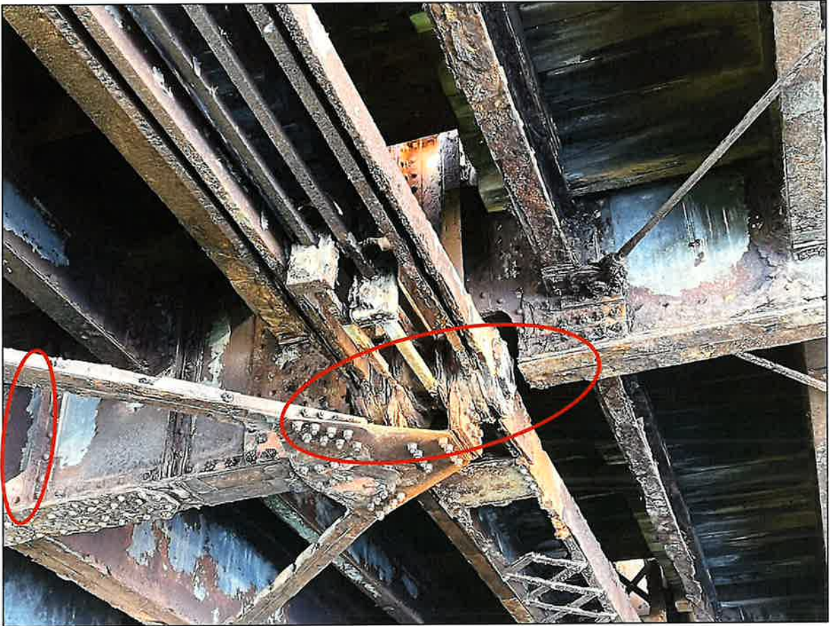
Photograph 9: Typical deterioration, section loss, and pack rust at pin connection (November, 2022).
