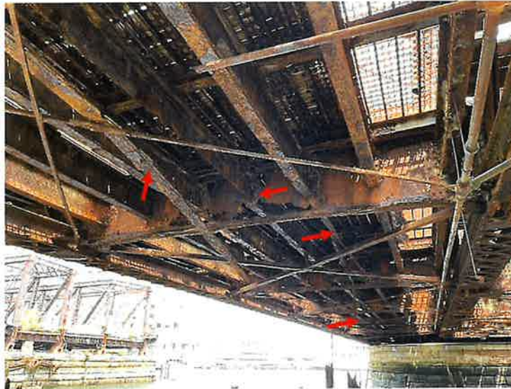
Photo 21: Swing Span, North Bay, Between Floorbeams FB10 and FB11 (Looking True North) Swing Span stringers typically have large rust holes however, these two stringers have failed webs and flanges, with hanging sections from the superstructure.
