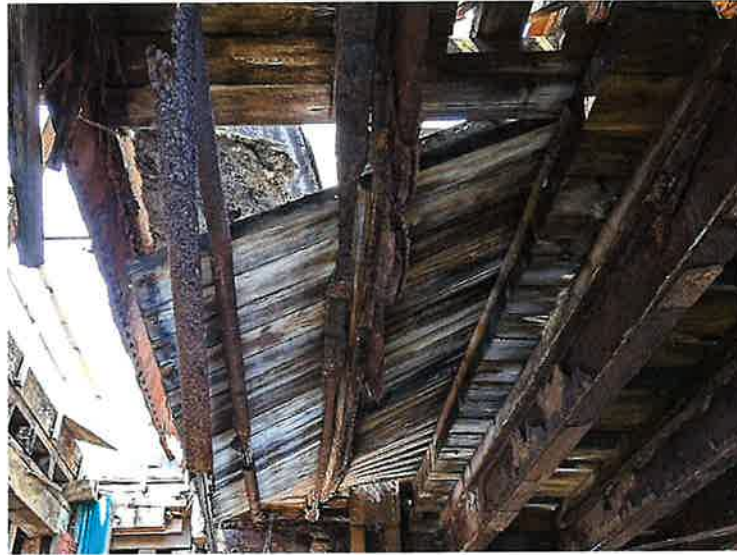
Photo 15: Approach Span 1, South Bay, Between Floorbeams FB1 and FB2, Deck and Sidewalk Stringers (Looking West)
