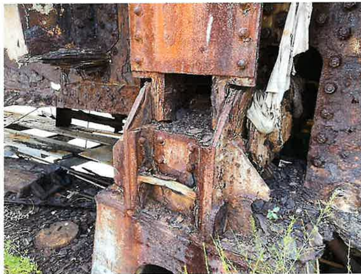
Photo 10: Approach Span 2, Pier 2, Center North Bearing L23 (Looking East) The pier bearings typically advanced deterioration with rust holes and pack rust.
