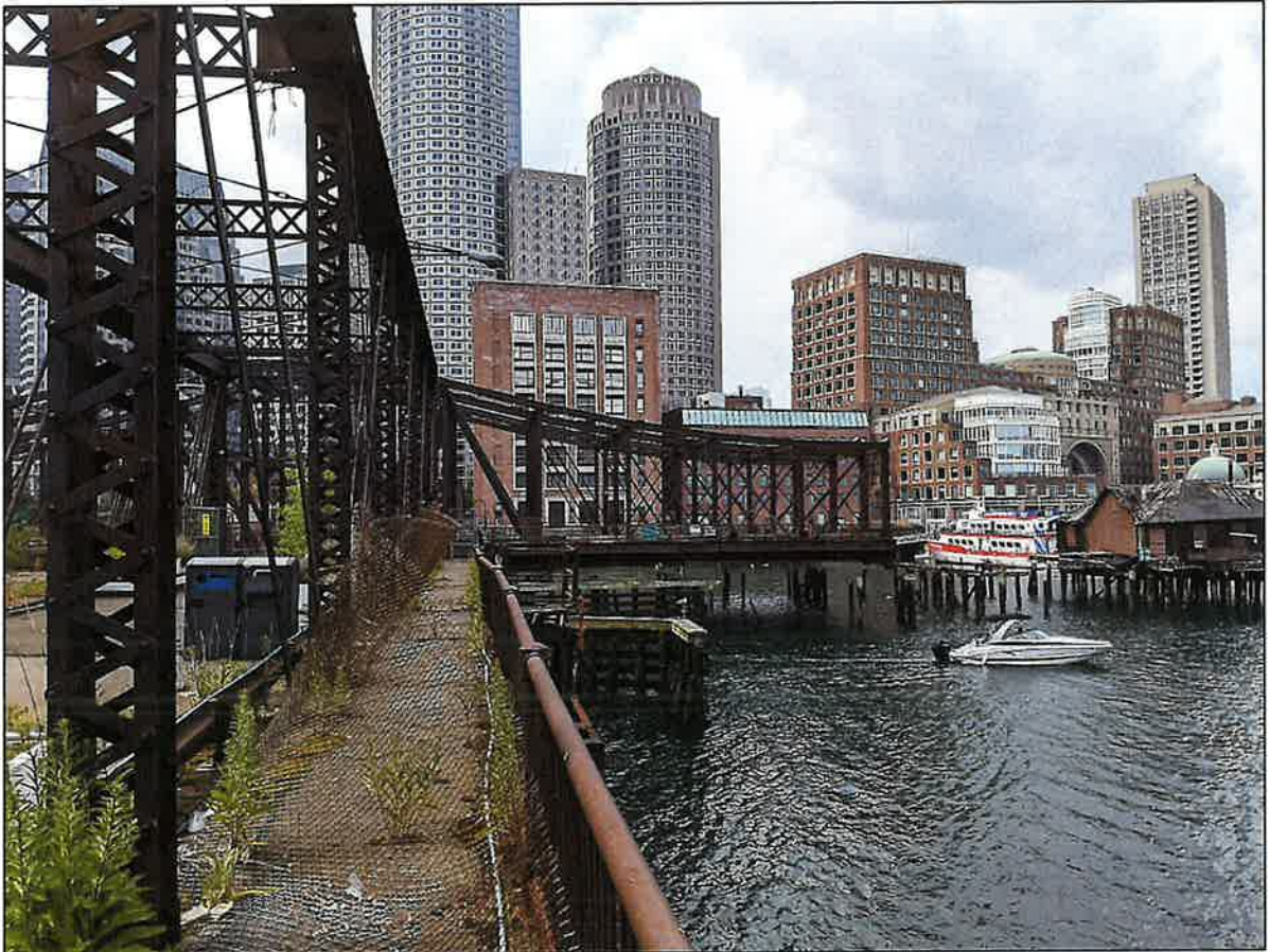
Photograph 3: View of open swing span from sidewalk on span 2, looking northwest. Note unsupported end of swing span (August, 2024).
