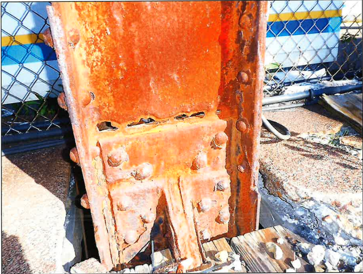
Photograph 8: Detail of typical deterioration of web on vertical member at deck level (November, 2022).
