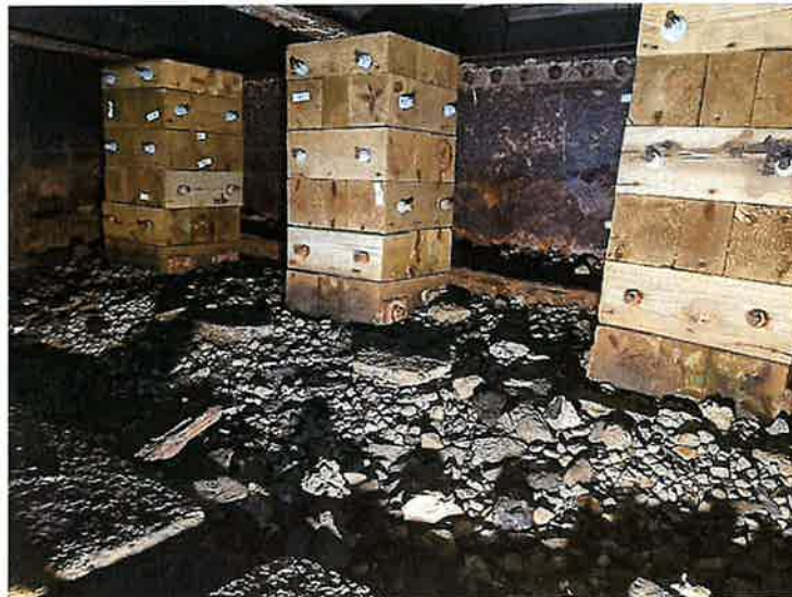
Photo 12: Approach Span 3, East Abutment, Timber Cribbing Bearings (Looking East) Approach Span 3 stringers and deck bear directly on the timber cribbing due to the failed abutment floorbeam.
