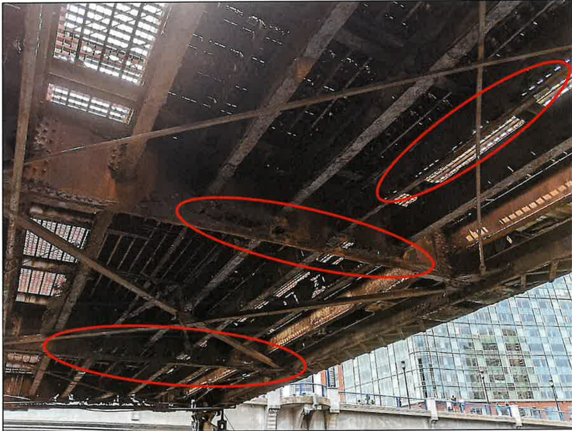
Photograph 5: Section loss at stringers and floor beams of swing span, looking southwest. (August, 2024).
