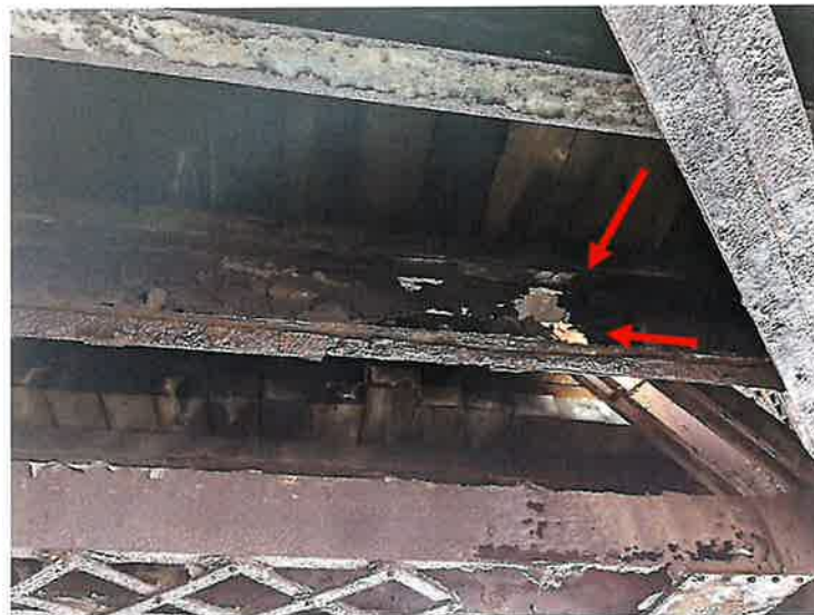
Photo 16: Approach Span 1, Center Bay, Between Floorbeams FB2 and FB3, Stringer 6 (Looking North)
