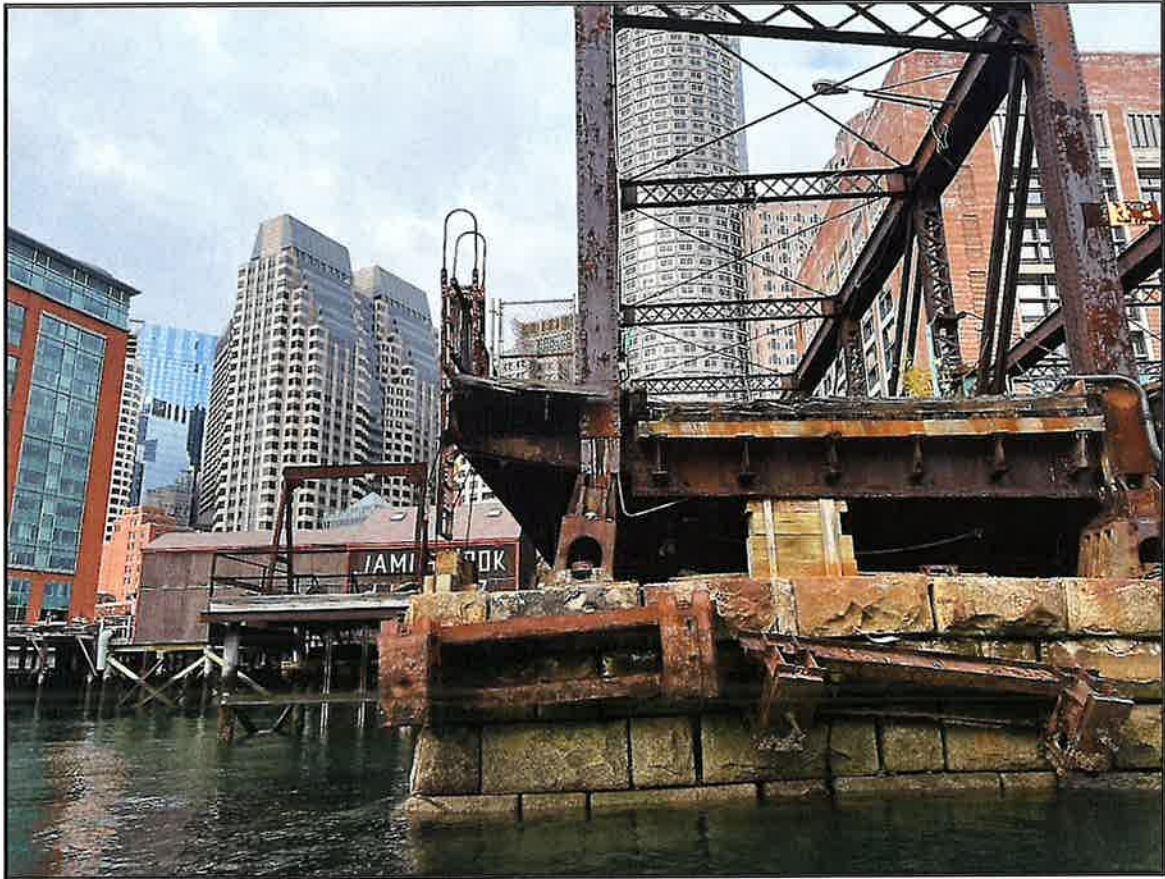
Photograph 7: Pier 1, looking west toward span 1 (westerly fixed, approach span). View of failed lagging repair and rotated bearing at pier (November, 2022).
