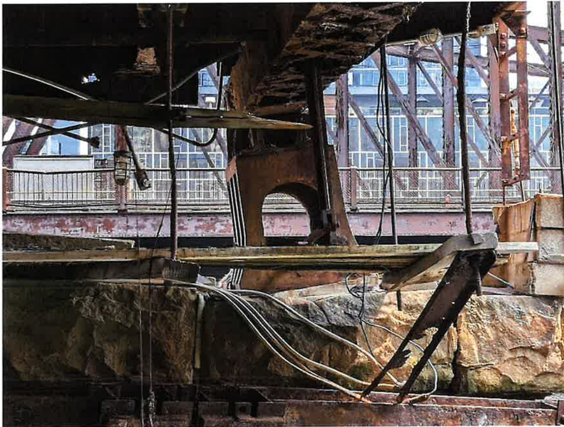
Photo 8. Approach Span 1, Pier 1, South Bearing L8 (Looking East) Settlement of the pier has caused the rotation of the bearing at A2S.
