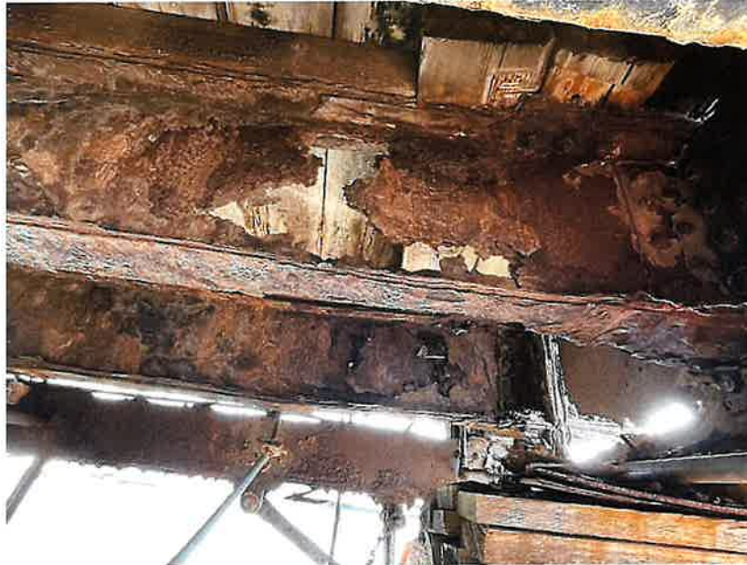
Photo 17: Approach Span 1, North Bay, Between Floorbeams FB7 and FB8, Stringer 5 (Looking East)
