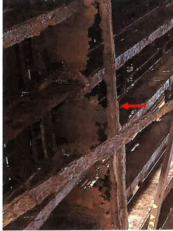
Swing Span, North Bay - Floorbeam FB10 (2024) *Advanced deterioration of existing rust hole since the 2017 inspection.
