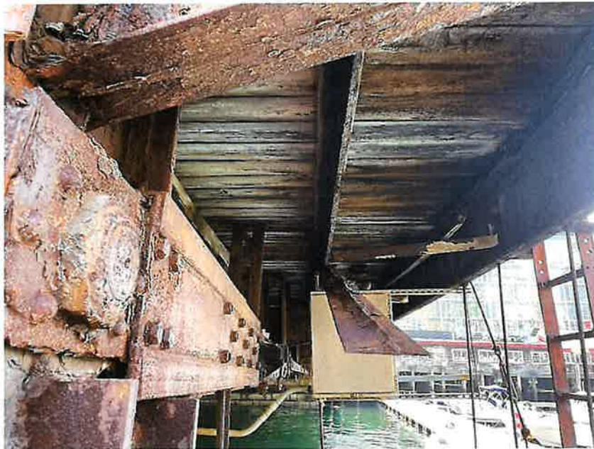
Photo 18: Approach Span 2, South Bay, Between Floorbeams FB23 and FB24, Stringer 2 (Looking East)
