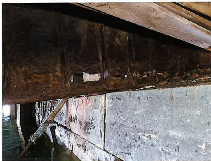
Photo 23: Approach Span 3. Girder P, Between Floorbeams FB5 and FB6 (Looking North) The approach fixed span girders typically have rust holes at the bottom of the webs and severely deteriorated bottom flanges.
