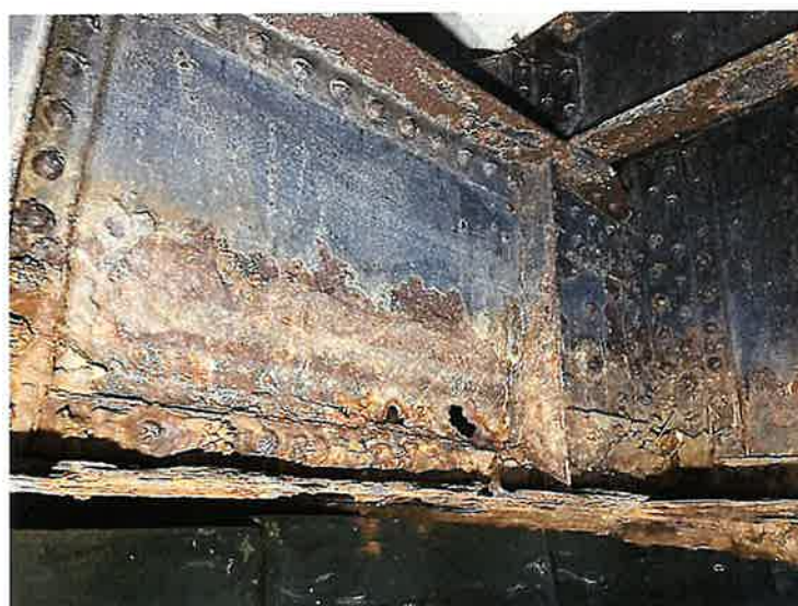
Photo 24: Approach Span 3. Floorbeam FB5, Between Girders GO and GP (Looking East) The approach fixed span interior floorbeams typically have small rust holes and section loss along the bottom of the web
