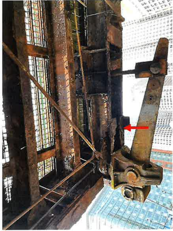
North Truss at L9L10 at L9 (2024) *Advanced deterioration of existing rust hole since the 2017 inspection.
