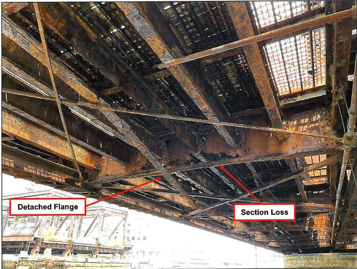
Photograph 4: Underside of swing span looking north. Note section loss in floor beam and detached flange from stringer (August, 2024).
