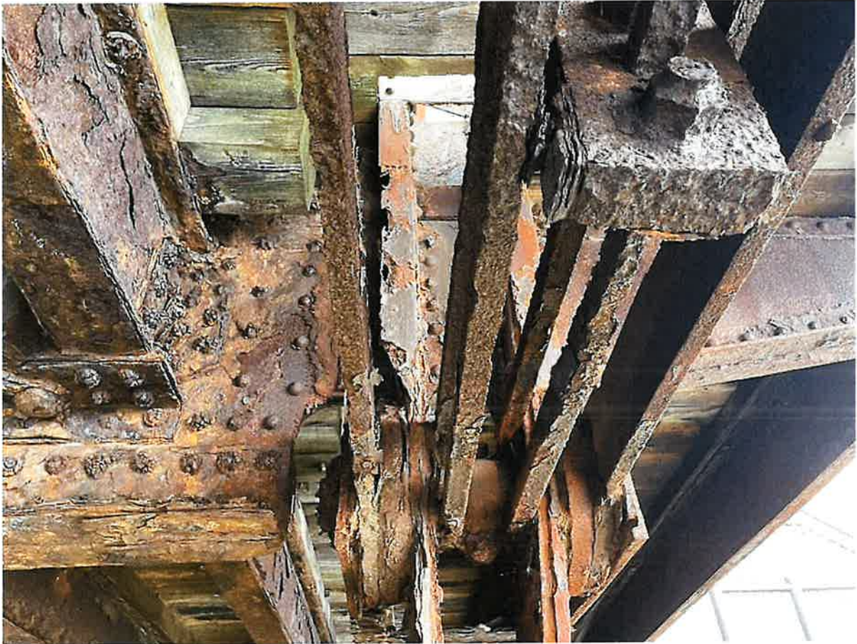
Photo 1. Span 1, North Truss, Lower Chord, L2-L3 (Looking West)
