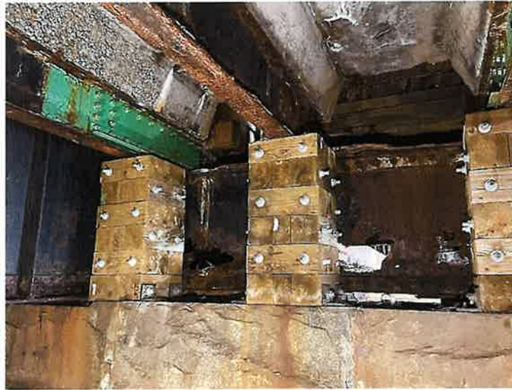
Photo 11: Approach Span 3, Pier 3, Timber Cribbing Bearings (Looking West) Approach Span 3 stringers and deck bear directly on the timber cribbing due to the failed pier floorbeam.
