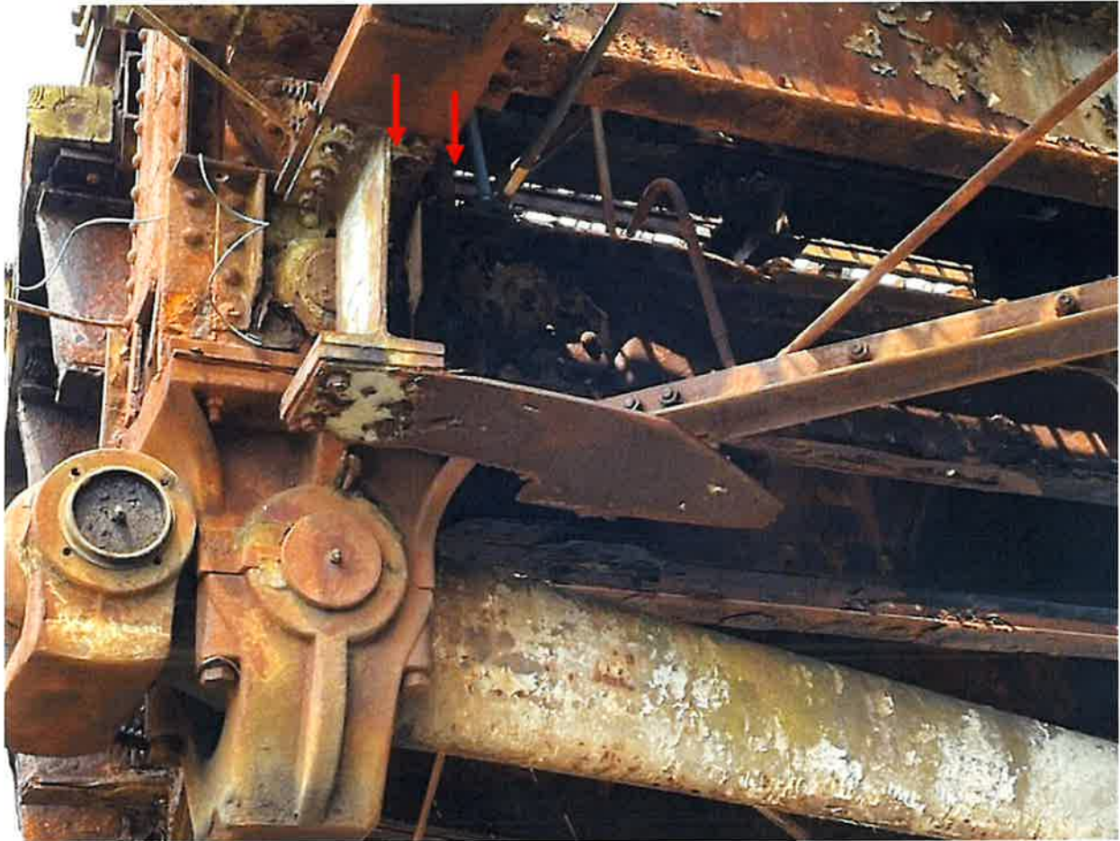
Photo 4. Span Swing, Center North Truss, Lower Chord, L9-L10 (Looking True North) The south channel web and top flange are buckled. Channel webs have up to 1/4" loss. The top and bottom flanges have rust holes
