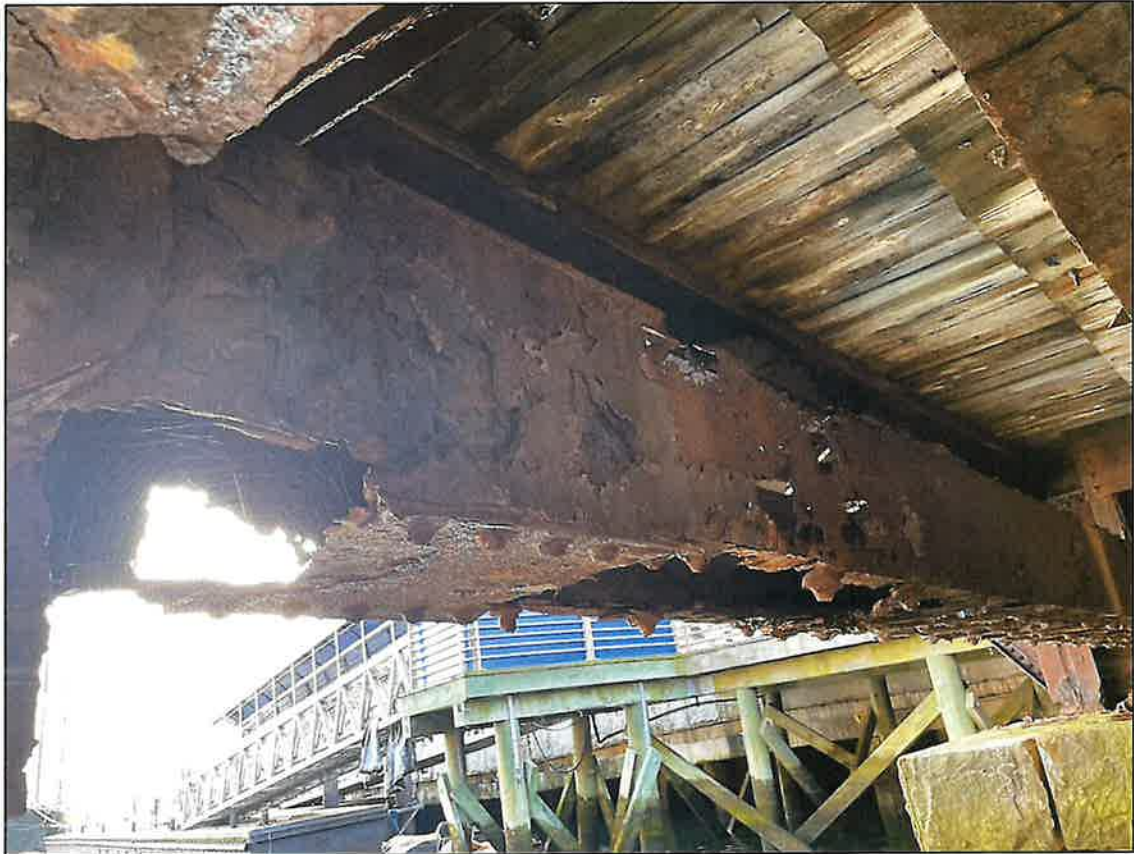
Photograph 6: Detail of stringer deterioration at span 2 (easterly fixed, approach span), and missing mortar from pier 3 looking northeast (August 2024).
