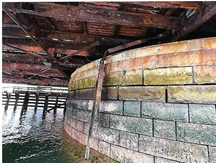
Photo 22: Swing Span, Center Bay, Between Floorbeams FB16 and FB17, Floor System Bracing (Looking True South)
