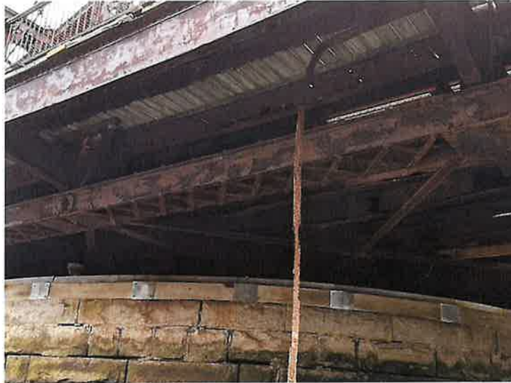
Photo 19: Swing Span, North Sidewalk Bay, East of Floorbeam FB14, Stringer 2 (Looking True Northeast)
